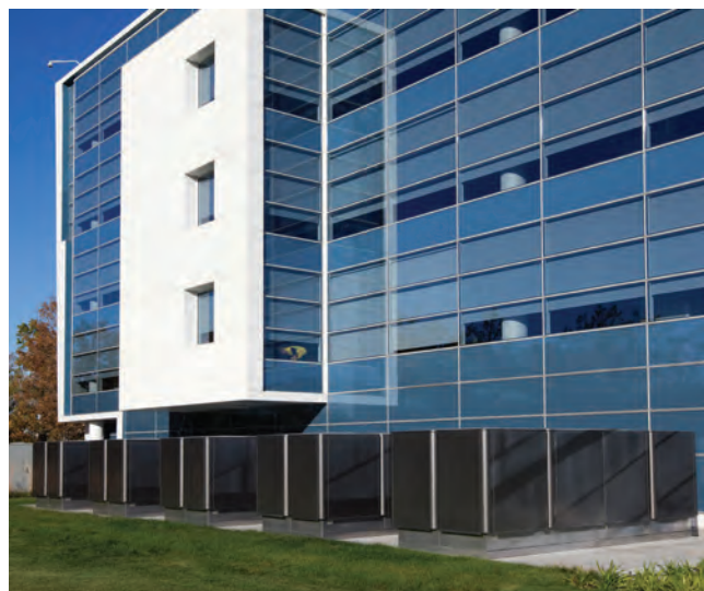
FIGURE 6: Bloom Energy Server Outdoor Installation
